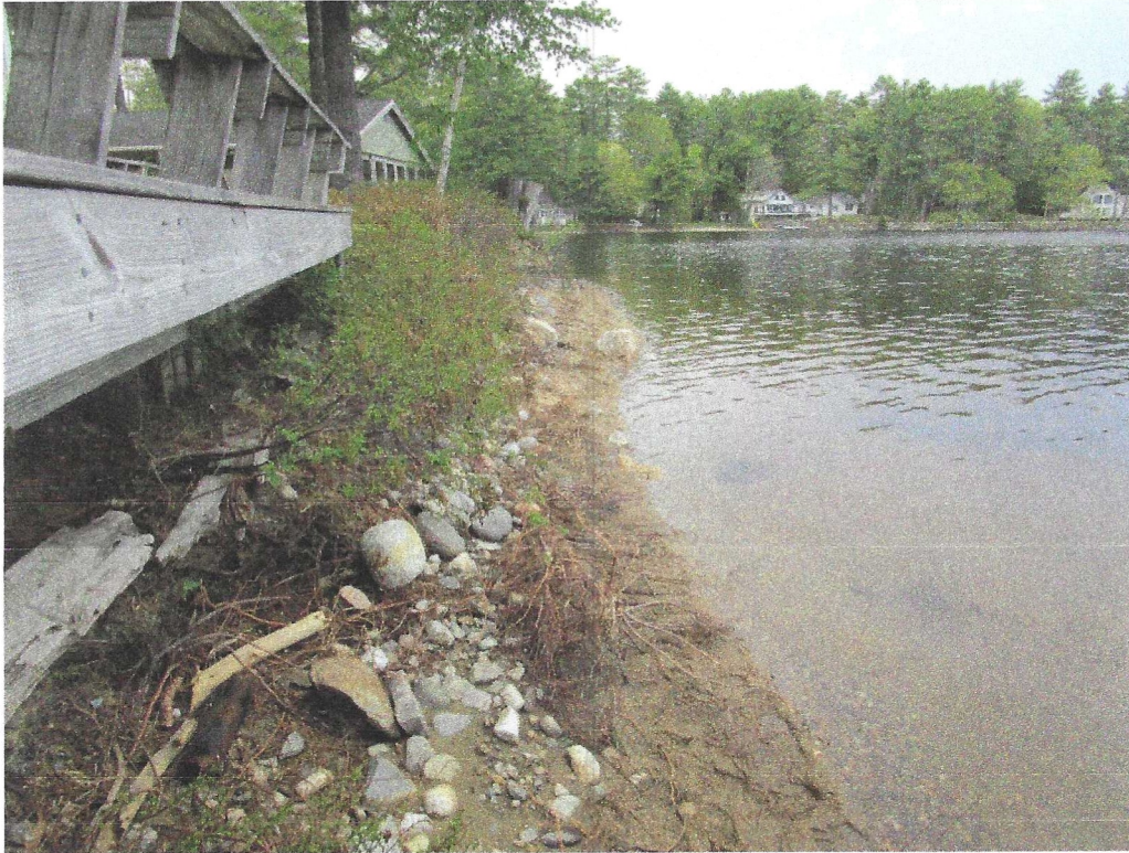
Photo 3. Close up view of the sweet fern shrubs on the shore that eroded from the bank during the heavy rain event on April 30, 2023.
