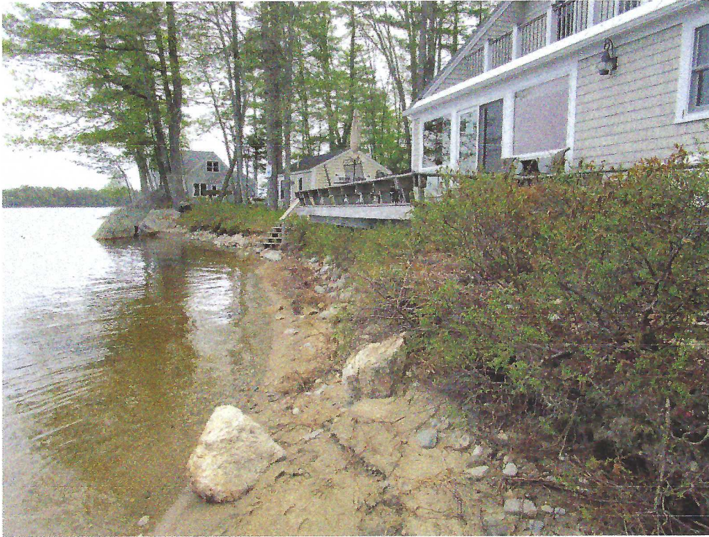
Photo 1. View looking south of the waterfront of Karen Johnson's property on Pemaquid Pond located at 108 Hoffses Beach Lane in Damariscotta, Maine after the heavy rains and erosion.
