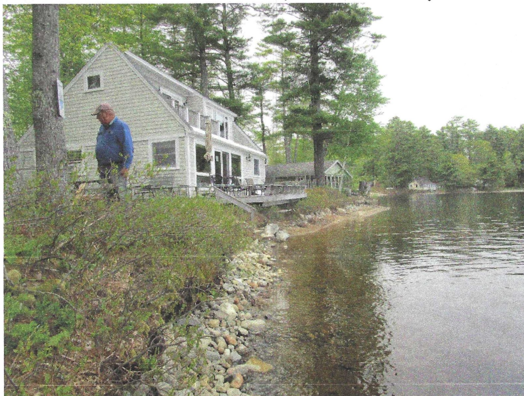
Photo 2. View looking north. The proposed riprap at the shore will extend 99' from the tree with the Lake Smart Award north to the property line with a 4' wide break at the footpath.
